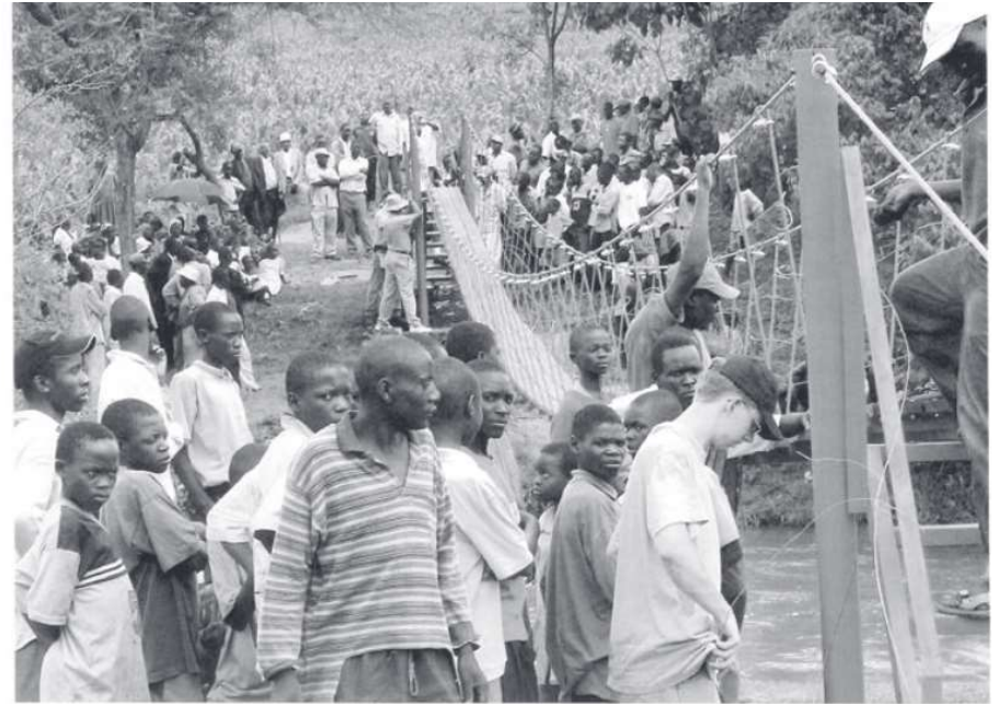
The bridge in Kenya built by Walter and students from Baylor saved villagers a twelve-mile round trip trek to get from one side of the river to the other.
